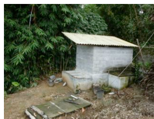
A toilet connected to a methane pit built with brick walls, cement floor and iron roof.
